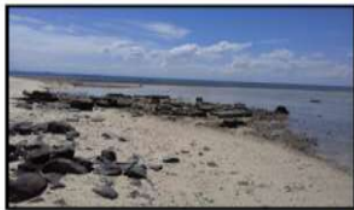
Figure 8. Ruins house that had been damaged by abrasion on the west season, in the southern part of the island.
